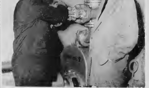
THE BEGINNING: J. J. Horigan, president, and O. S. Mingu, general manager, prepare to open the valve discharge which set in motion the new refueling pump for 100 octane gasoline at Dakota Field. The occasion, which took place January 24, was attended by officials of Esso Standard Oil S.A., on visit here.
